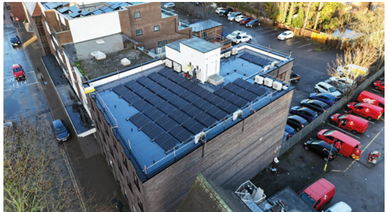
Solar panels are expected to meet around 25% of the building's annual electrical demand
