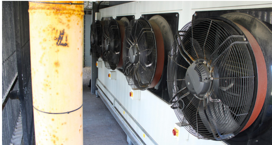
One of four sets of ASHP evaporators next to a gas pipe at the university college case study
