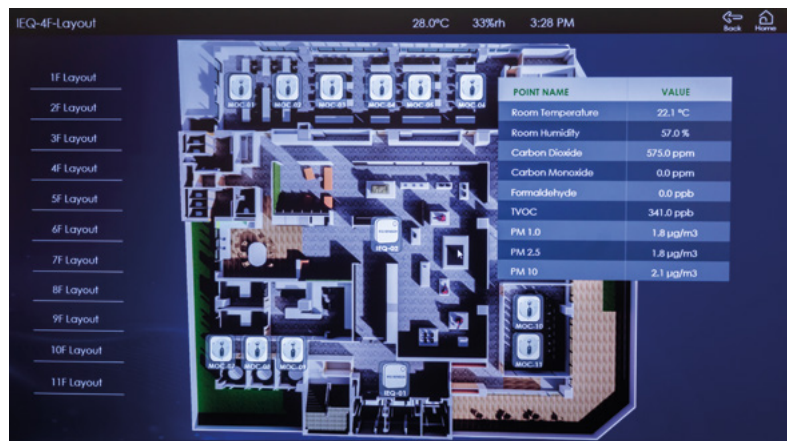
BMS dashboard showing real-time indoor environmental quality readings
