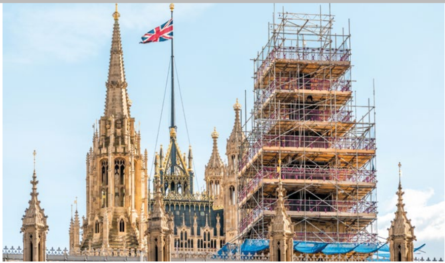
An ultimate test of the 'restore vs retrofit' dilemma, the ongoing work at the Houses of Parliament is tackling decades of decay by replacing services within one of the world's most complex heritage sites
