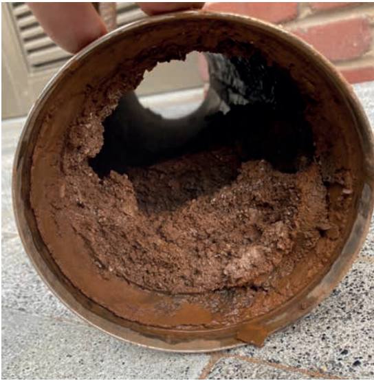
Figure 1: A 40µm filter basket from a reaction tank (as in Figure 3) that was removed shortly after installation into a new-build system
