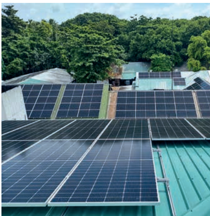
The new solar installation at the back-of-house facilities at the Soneva Jani luxury eco resort in the Maldives
