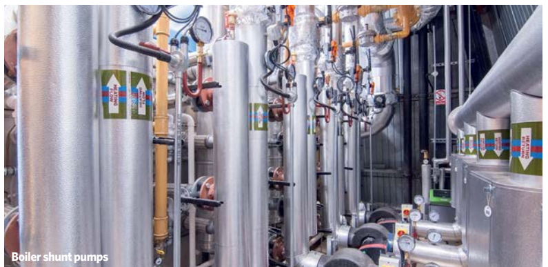
Boiler shunt pumps
