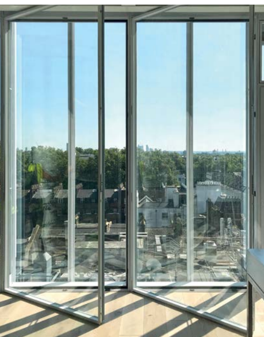
Internal doors in the inner skin of the façade allow for cavity cleaning and maintenance
