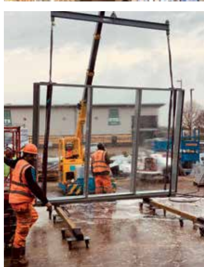
More than 3,500m 2 of façade panels were dismantled and refurbished during the revamp of 1 Triton Square
