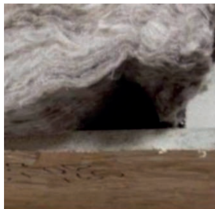
Defective workmanship showing insulation gaps
