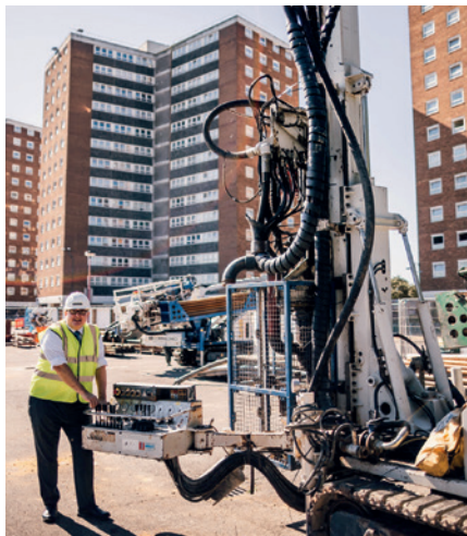
The new heat pumps will replace 273 storage heaters
