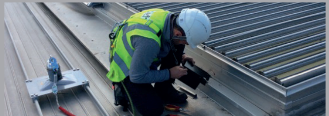
Product testing inspection underway, prior to the commissioning of a newly installed smoke control system.
